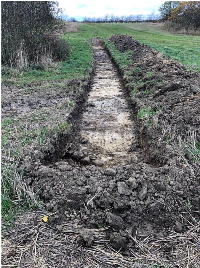
Image 4. Excavation of the ground to look for drainage pipes immediately north of the pond in area 5.
